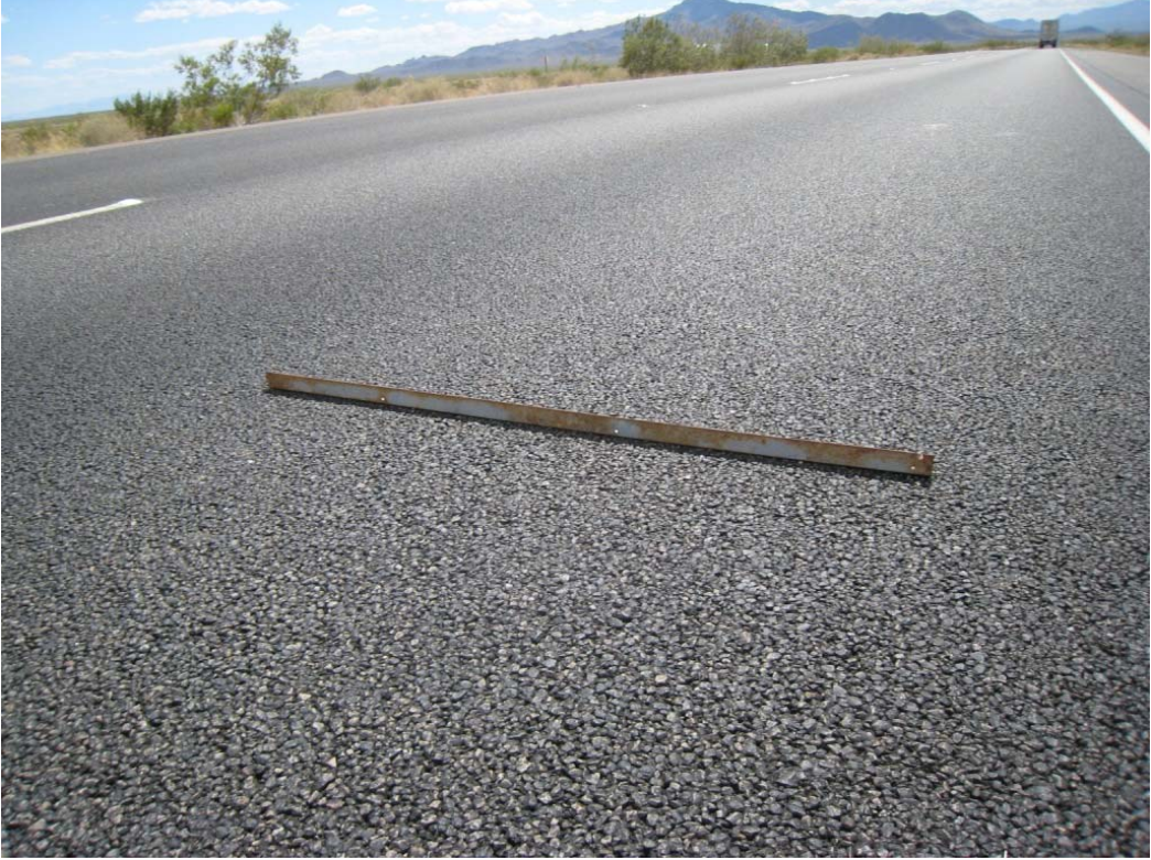
PM; Zero rut depth at start of PM Test Section at 0'
